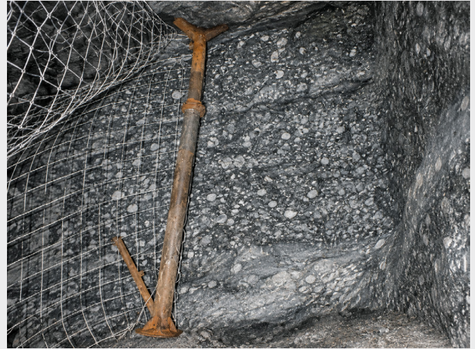
Figure 6: Post TARP - Reef fully exposed and face not overhanging.
