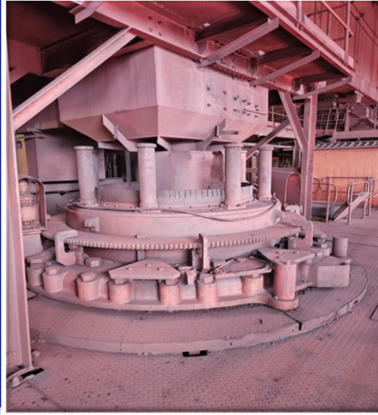
Crusher Unit – Feeder Level
