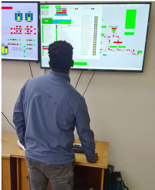
Figure 1: Team viewing the Conveyor Belt Overview System which indicates the operation’s underground conveyor belt system and the location of the CBAT and CRTM System. Source: Seriti Khutala Colliery
