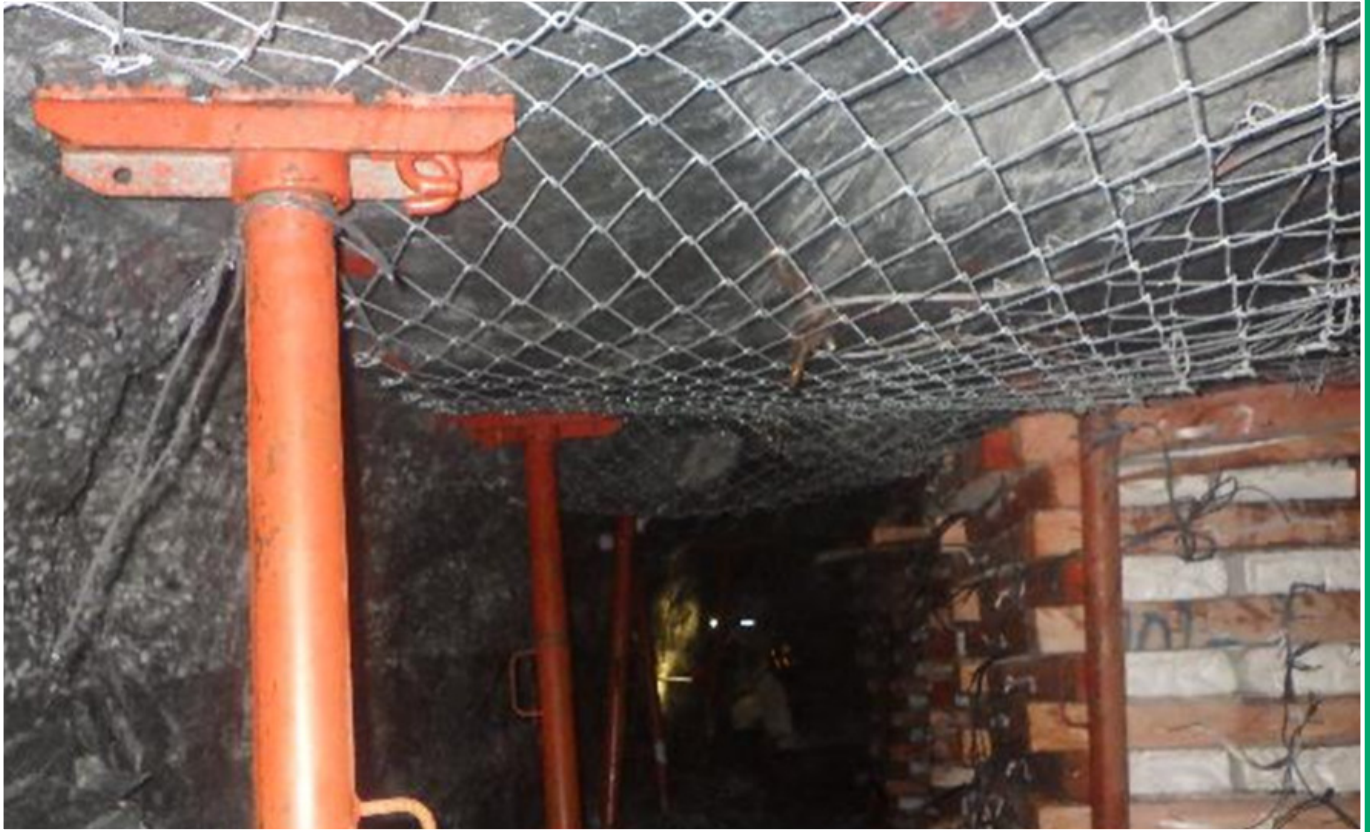
Figure 2: Mesh pinned against the hanging wall with camlock jacks and bolts
