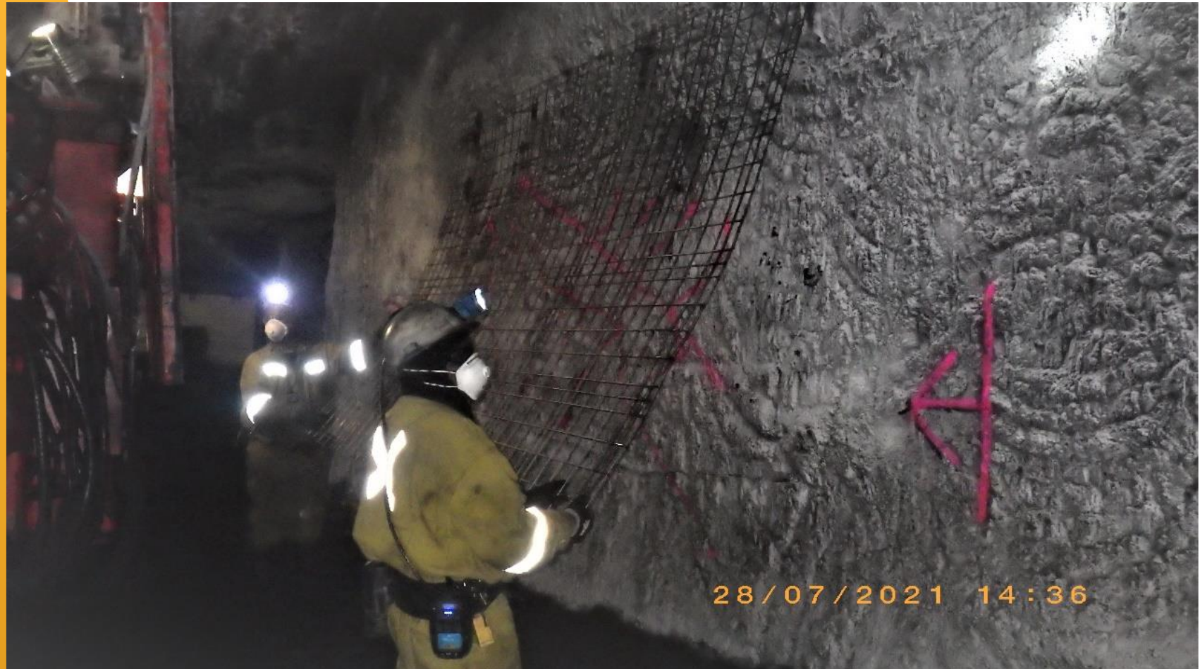
Image 7: Placing the mesh sheet onto the Z-Hooks – Note the distance between people and sidewall.
