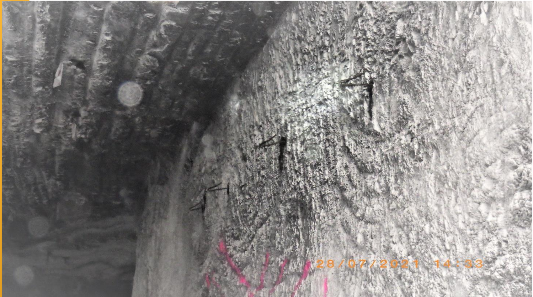
Image 6: 4 x Z-Hooks installed – Note the positions: above the “unstable” area being meshed.
