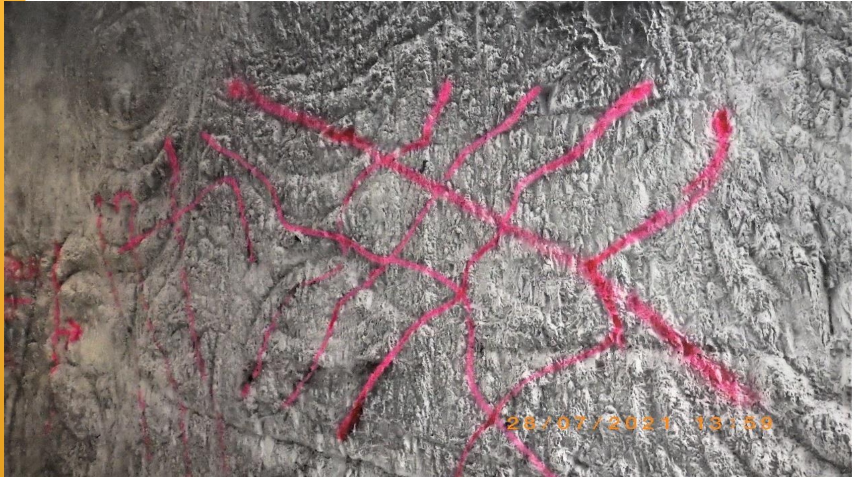
Image 1: Identification of the area and marking of fictitious sidewall slips.
